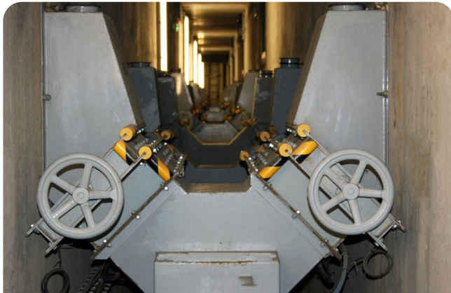
Valves under cells
